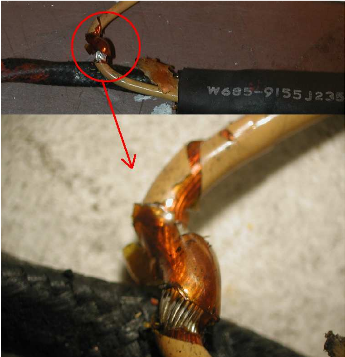
Figure 1. Harness H16DW685-9155. Breach of wire insulation down to the conductor.
