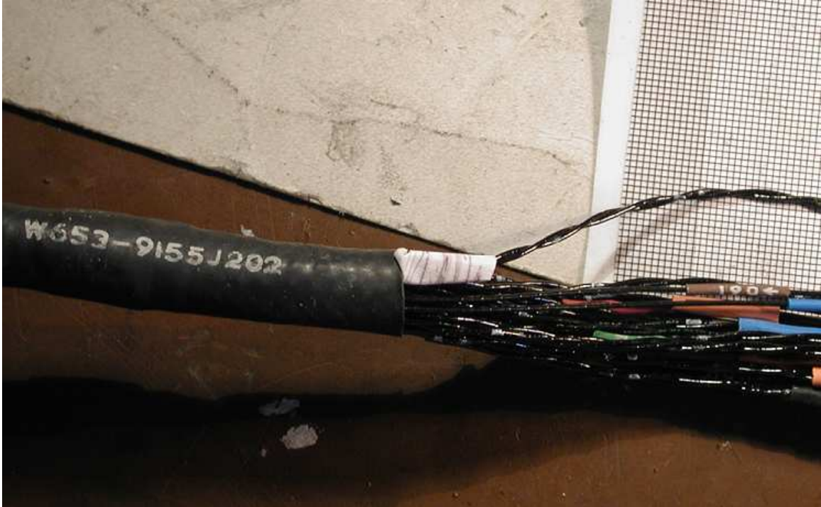
Figure C-7: Harness: H16DW653, wire224-1. Break in 24 gauge wire. Background grid scale 1mm x 1mm.
