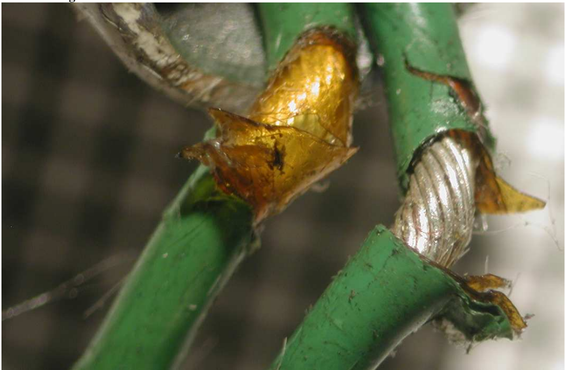
Figure C-4: Harness H16DW606-21 (a). Wire 2 has exposed conductor. Damage to the insulation of wire 1.
