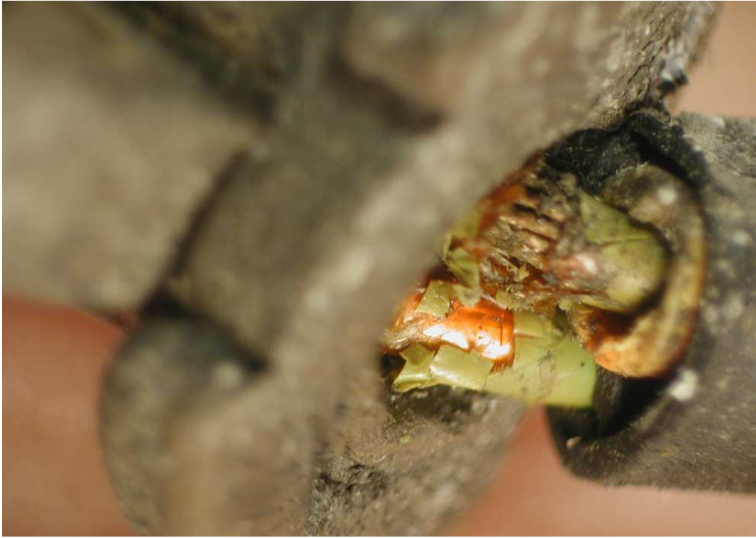
Figure C-9: Harness: H16DW693-21. Wires coming out of a conduit with multiple breaches to conductor.
