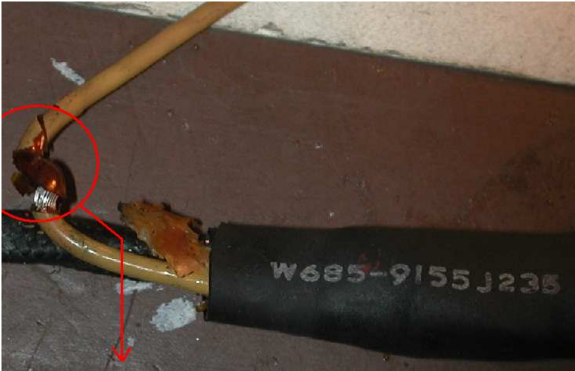
Figure C-1: Photo: Harness: H16DW685-23. Conductor exposed
